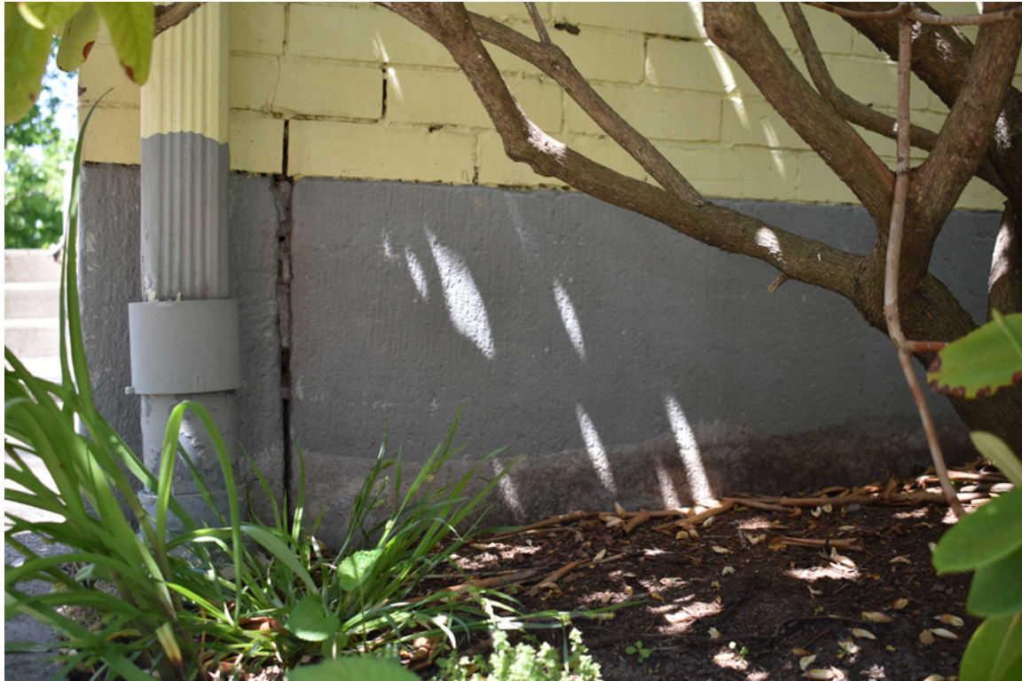
Figure 7. Daniel Withington House, hammerhead granite foundation detail, looking northwest (The Public Archaeology Laboratory, Inc. 2021).
